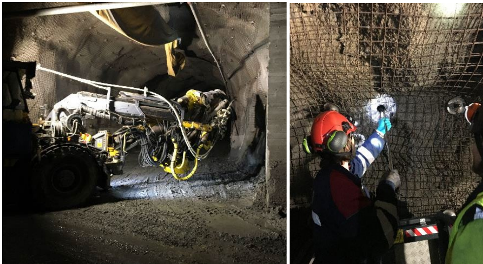
Figure A: Drilling and installation of 3D load cells for stress measurements
