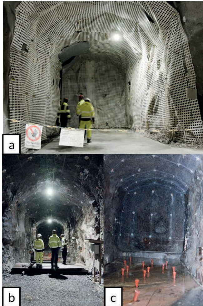
Figure 10. Site inspection at ~400 m: a) site TAS05 b) site TAS04 general view c) site TAS04 water ingress on tunnel floor.
