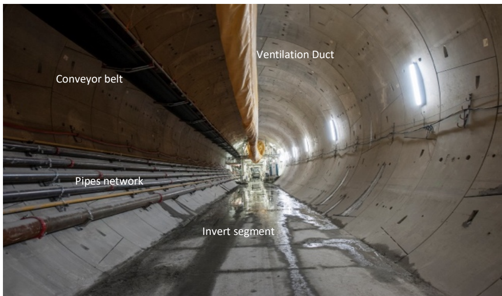
Figure 4. Systems in the TBM tunnels
